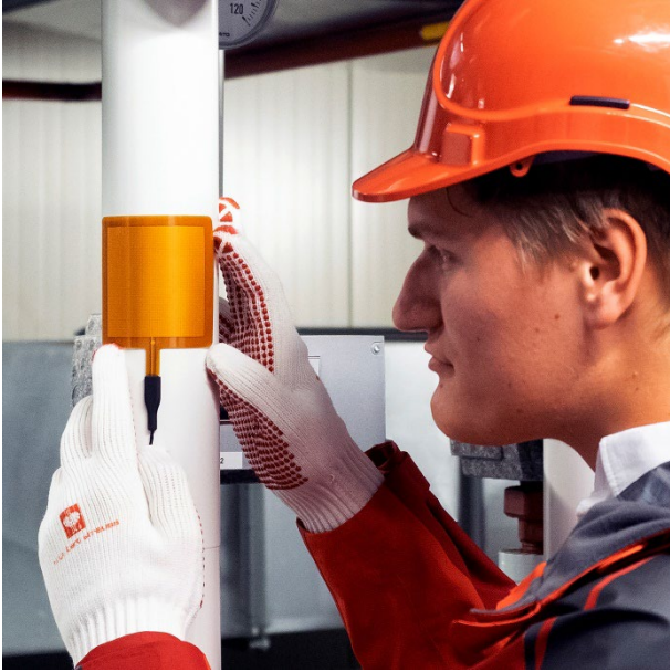
Figure 2 FHF05-85X85 being installed to measure heat flux on a pipe.
